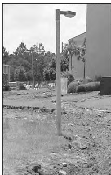
Annie Johnson / The Spectator Library construction re-routes traffic The main footbridge to the Fine Arts building is now also blocked off.
