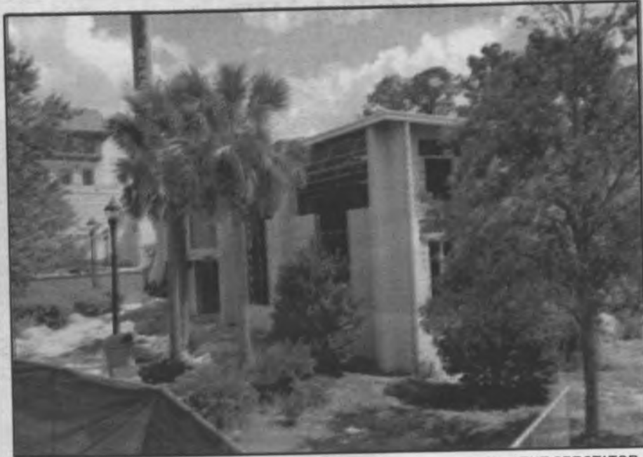
Bryce Ethridge/ THE SPECTATOR VSU began Pine Hall's renovations earlier this summer and plans to finish construction spring 2018.
