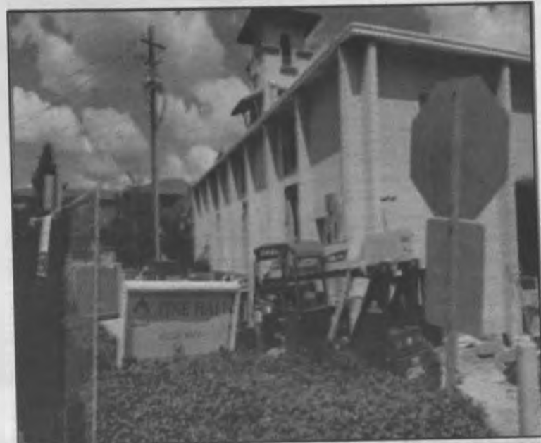
Bryce Ethridge/ THE SPECTATOR The construction for the renovation of Pine Hall has displaced much of the IT department.
