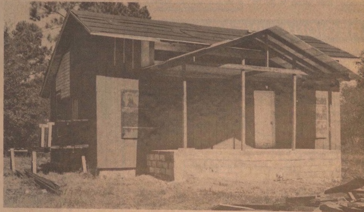
House On Hedgewood Circle Caused Neighborhood Residents To Ask City Code Be Changed
