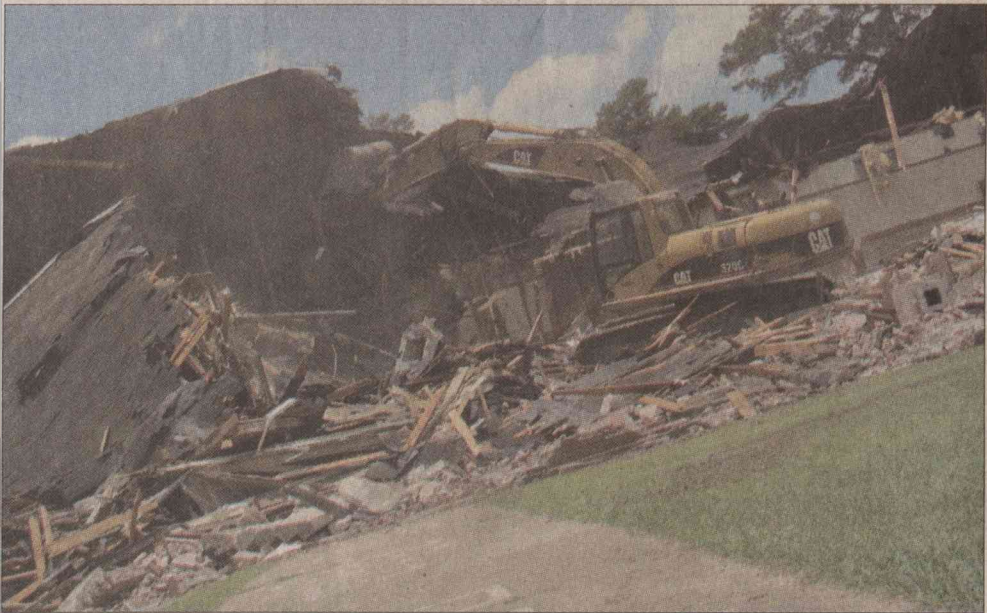
NICK GERALD of Calmart, Inc., made quick work of razing this 1938 building on the Southside Elementary School campus. Work began Tuesday morning knocking down the brick walls and shortly after the noon hour the roof began to come down.
