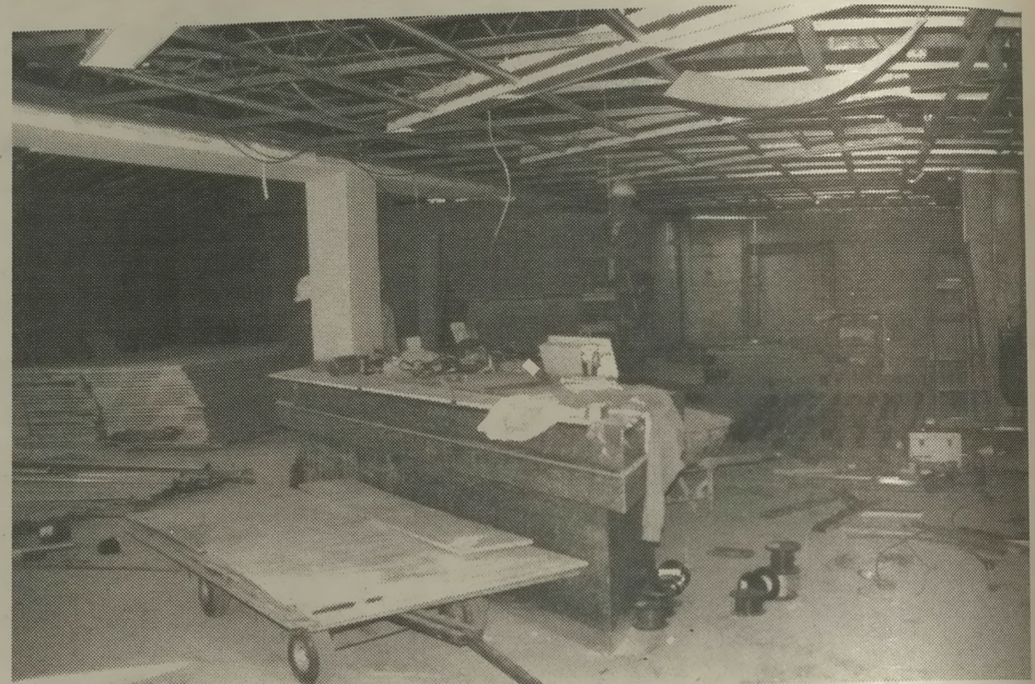
Interior view of construction in the new Annette Howell Turner Center for the Arts.
