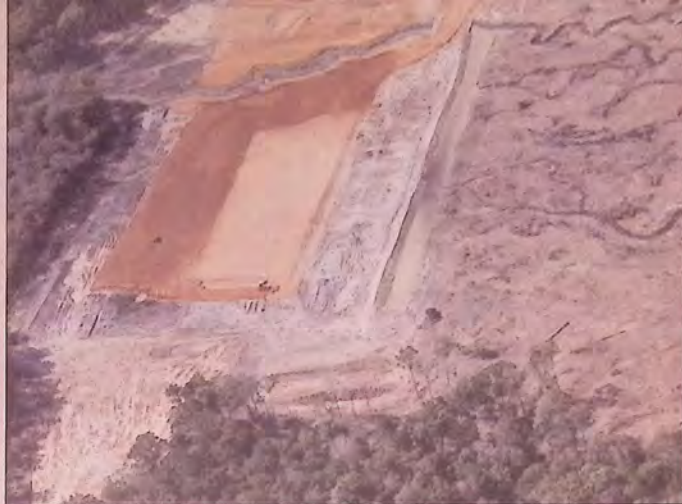
GOING DOWN... Crews have excavated this huge section of the dam site as crews prepare to pour the slurry wall. When the wall is poured as many as 25 concrete trucks a day will be in and out of the lake site, officials say.
