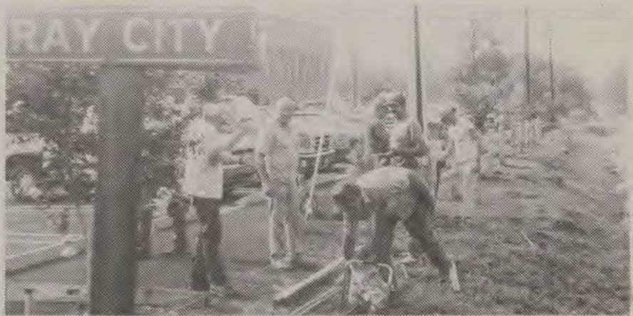
Workers assemble split rail fence as part of the beautification project along Paralled Street parking lot.
