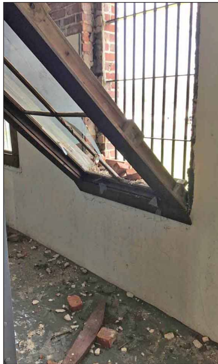
The Old County Jail was really beat up by Hurricane Helene in September 2024, as evidenced by the two window frames and brick work blown out completely.
