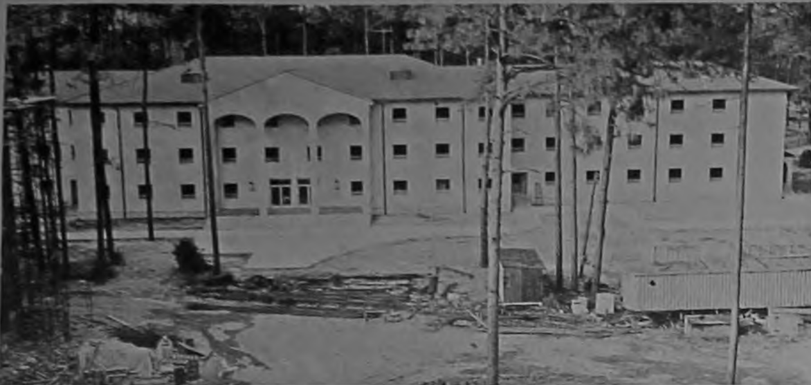
Construction on two new residence halls for women at Valdosta State College continues at a rapid pace. Finishing touches are being added to Georgia Hall (in background), a 200-bed residence hall. Langdale Hall, left, is rapidly taking shape, and the 500-bed, five-story structure will be ready for occupancy fall quarter.
