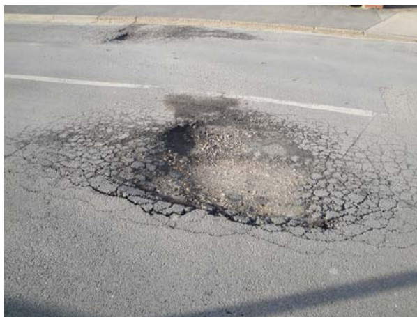
Figure 13.14 Thermal stress contributes to the formation of potholes. (credit: Editor5807, Wikimedia Commons)
