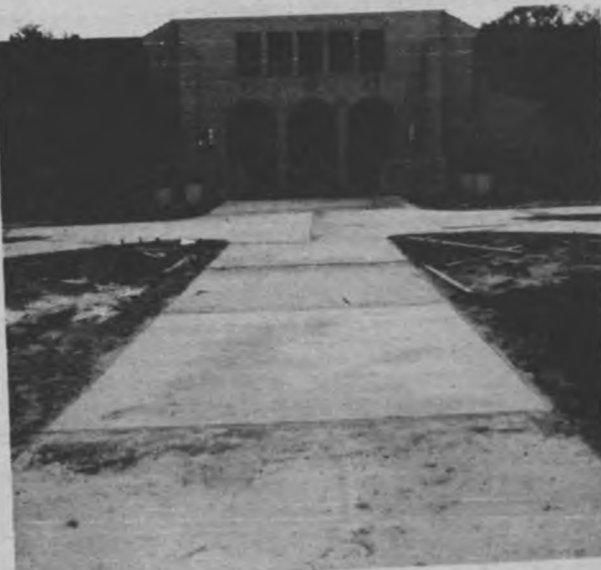
The rains may come, but at last the sidewalks leading to the cafeteria have been completed; so students no longer have to wade to dinner.
