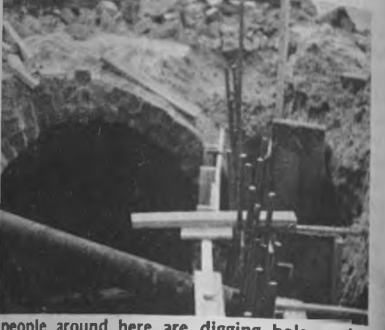
people around here are digging holes and r roads are busily caving in, as evidenced by reet. Repair is, and has been underway for of Patterson will have to be torn up in order
