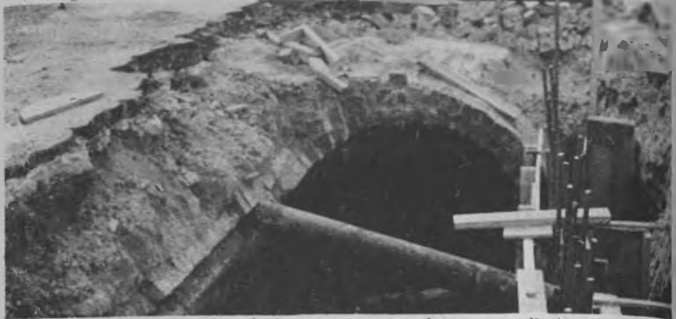
While the majority of the people around here are digging holes and building roads, some of the older roads are busily caving in, as evidenced by this large cave-in on Patterson Street. Repair is, and has been underway for some time. It is not known if all of Patterson will have to be torn up in order to initiate proper repair.
