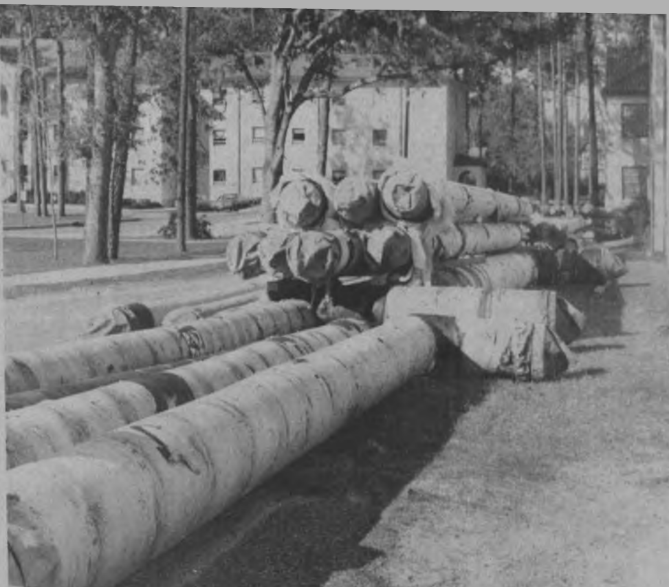
This summer will see this pile of steam pipes and others like it put underground at VSC as the campus renovation continues.
