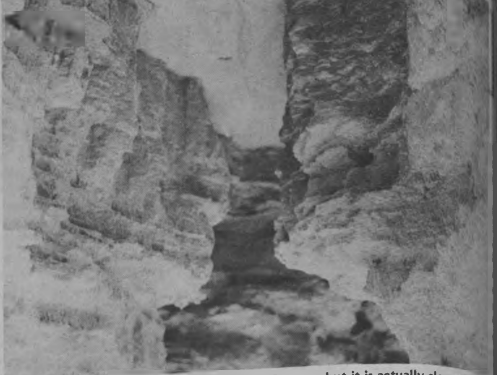
This may look like the Little Grand Canyon, but it is actually close-ups of the many washed-out areas on Baytree and around the Fine Arts Building. The Summer quarter at VSC will probably be even muddier when the underground electrical system and steam pipes are installed. Yes, Ladies and Gentlemen, happy mud fights days are on their way.
