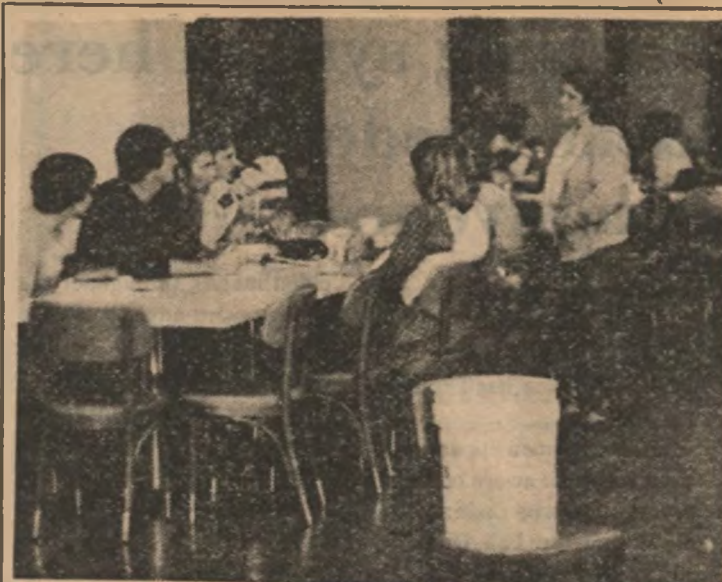
As the monsoon season approaches, the cafeteria crew prepares by breaking out the water buckets to catch the onslaught of rain drops from the leaky roof.
