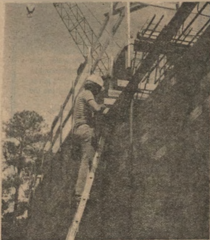
Construction worker Greg Evans adds some brickwork to the new gym. The complex is about a month ahead of schedule.
