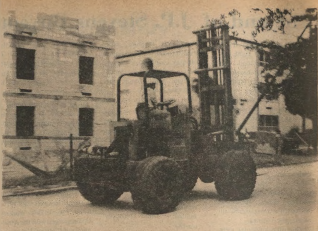
When not laying brick, setting forms, or installing windows, workman on the new Converse Hall apartment complex take turns driving the forklift around the building, as seen in this photo.
