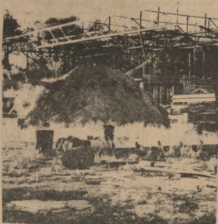
The area around the construction site is strewn with beams, metal strips and other assorted scrap.
