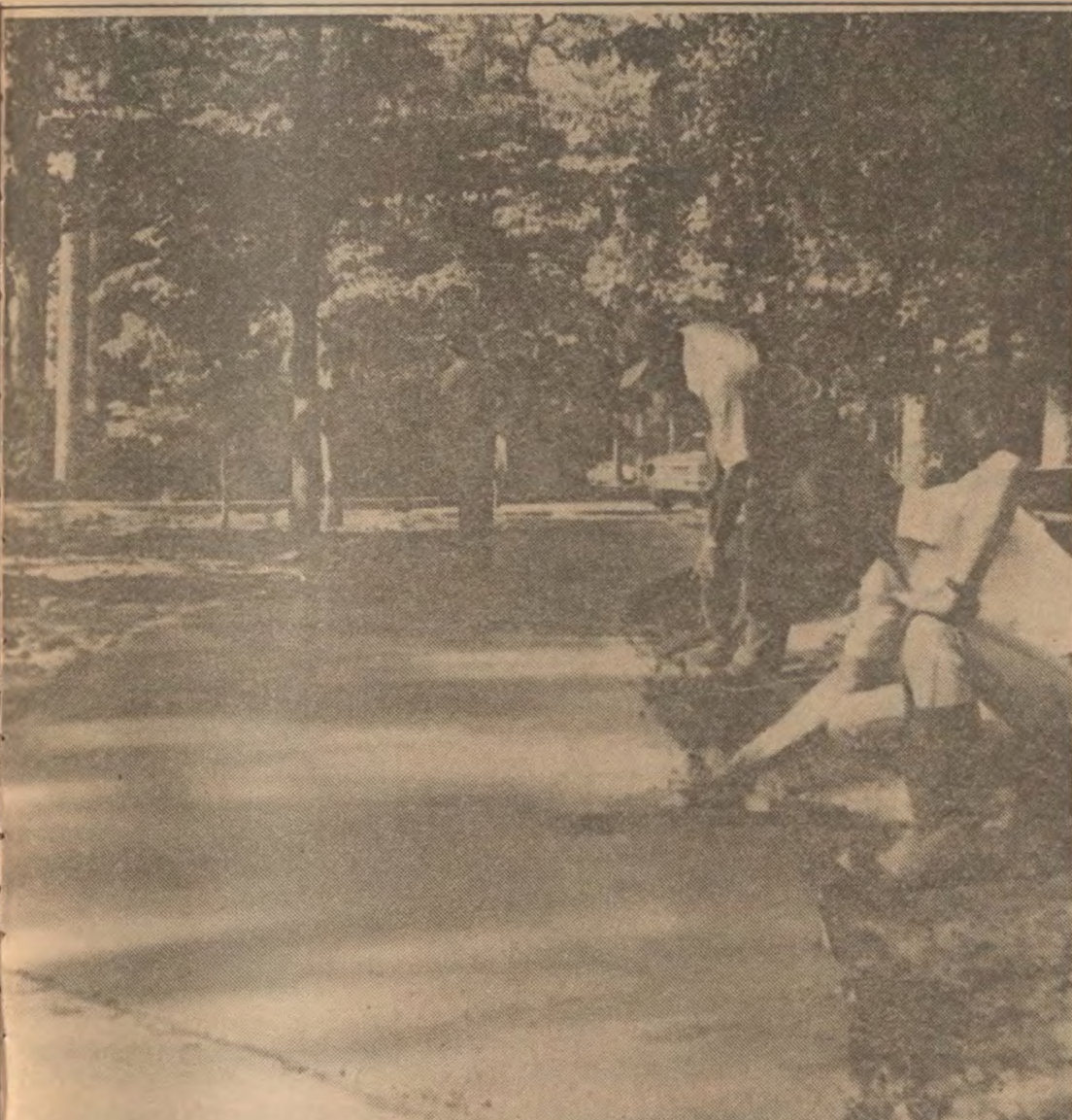
For students who dislike walking in the mud, a new section of sidewalk near Georgia Hall has just been completed.
