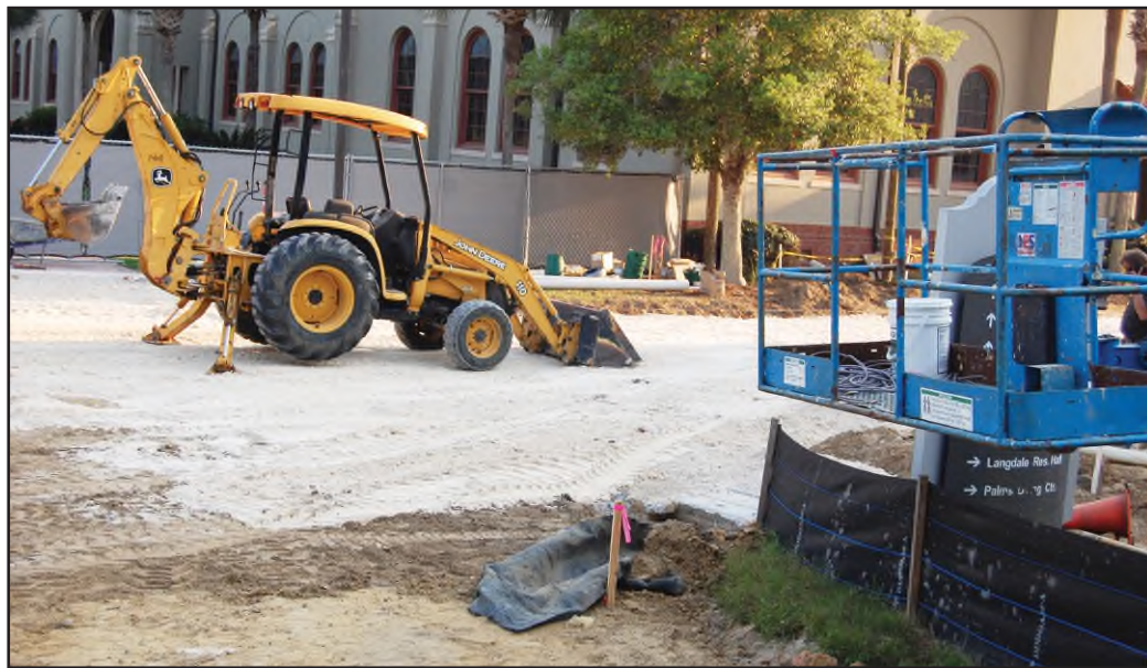
Construction equipment sits outside of Bailey Science Center. The addition to the building is scheduled to be completed on June 1.
