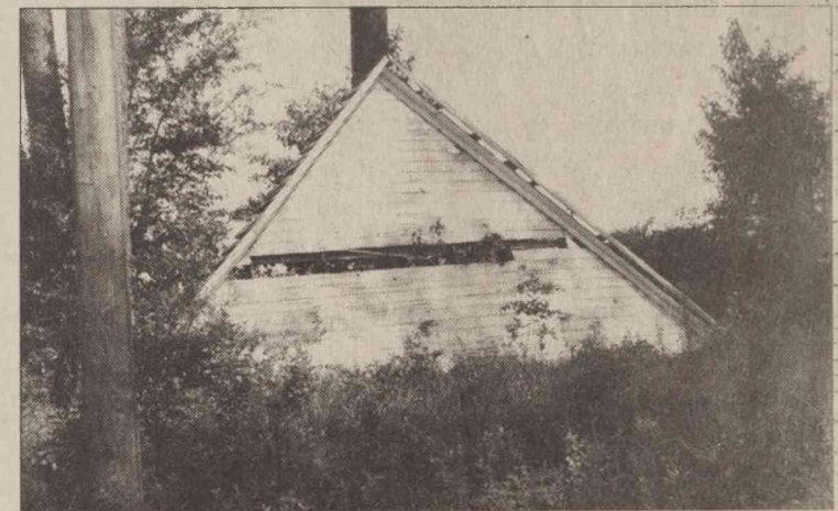
NOW COMPLETELY TOPLESS, the Pine Park Community Center building has its roof removed in preparation for its long journey to Graceville, Fla.
