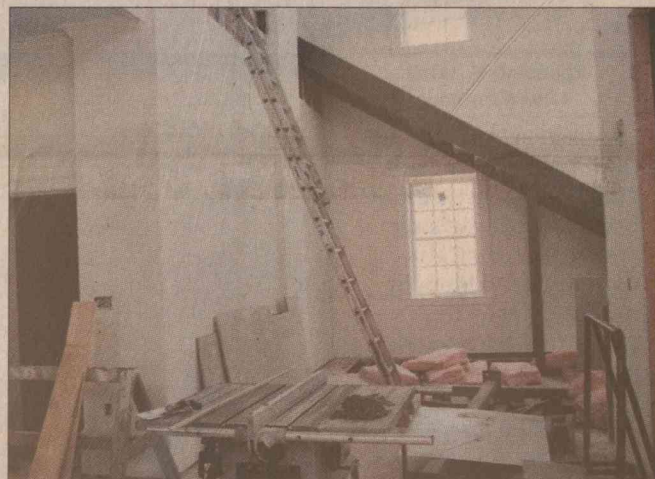
WORK IS PROGRESSING in the lobby of the newly renovated Southside auditorium. A staircase in the background leads from the lower level to the balcony. An identical staircase is located on the opposite side of the building. At left is an elevator shaft for a new elevator that will provide access to the balcony level.
