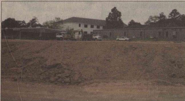
CONSTRUCTION AT SOUTHSIDE for the new administrative building and classrooms is expected to ramp up in the next few weeks.
