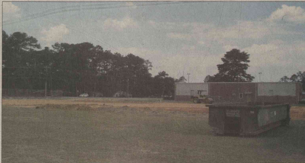
SITE WORK is underway for the new College and Career Academy facility being built just south of the NJROTC building. A groundbreaking ceremony featuring Lt. Governor Casey Cagle is tentatively set for Thursday, June 23 at 1:30 p.m.
