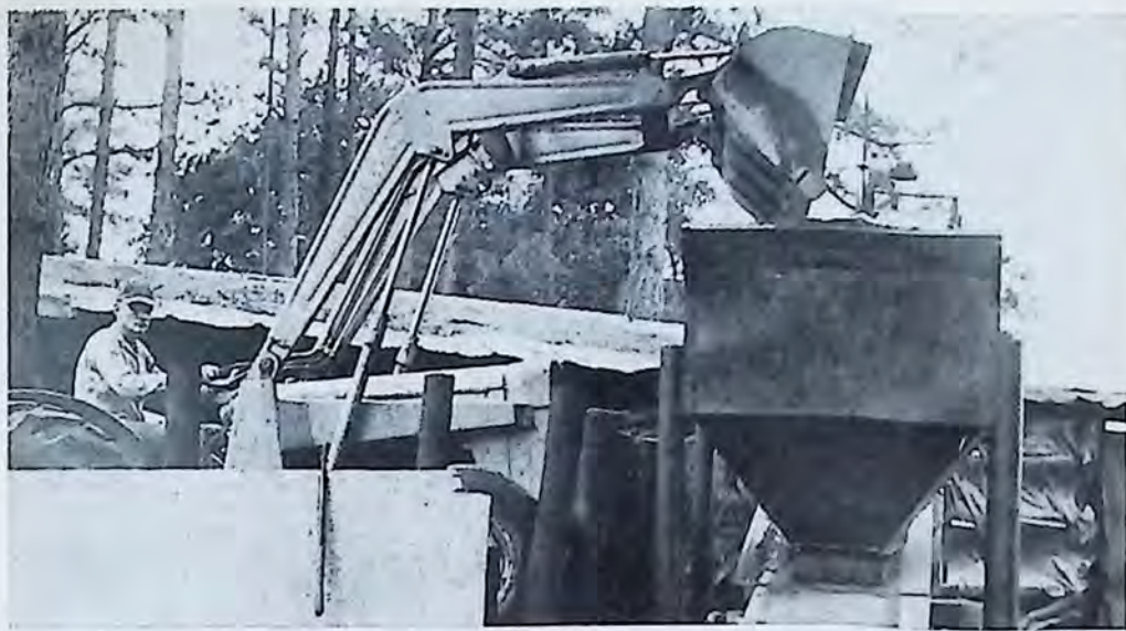
Tractor-mounted front end loader (with a half-yard capacity) mixes the canning mix on a concrete slab, then moves its load up a ramp and dumps it into the hopper . . .
